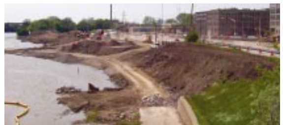
Construction continues on North Bank Park at Neil Avenue and Spring Street.
