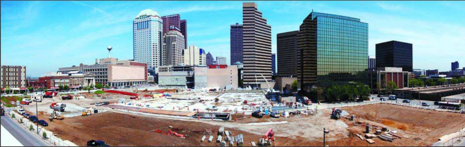
COURTNEY HERGESHEIMER DISPATCH PHOTOS A panoramic view of the construction at Columbus Commons park Downtown was created by "stitching" together several photos with computer software.
